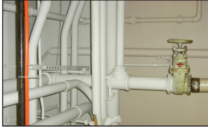
Piping and plumbing systems
