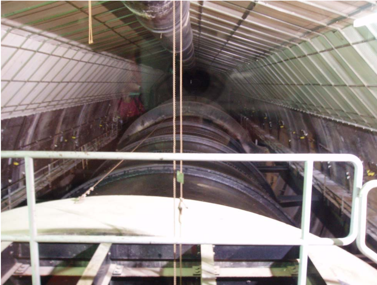
Hoover Dam Penstock
